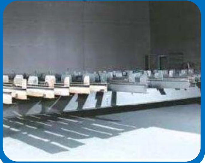
SHOT BLAST ROOM
