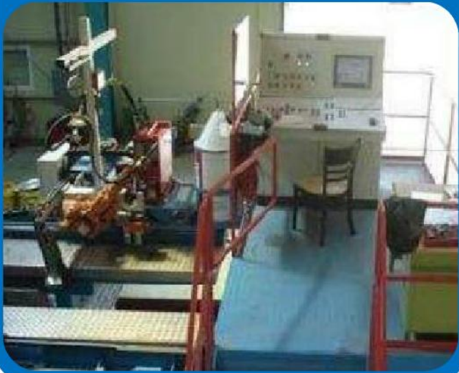
Main control booth
