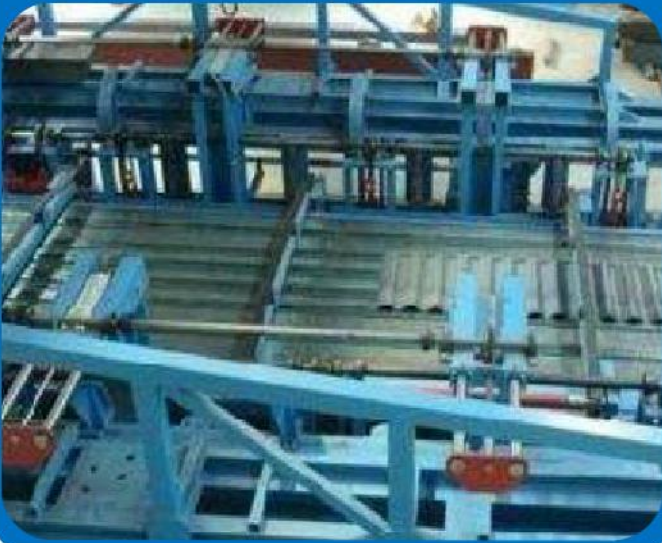
Corrugater web conveyor
